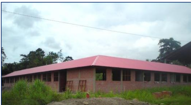
New Classrooms for the San Antonio School. ceilings for the new classrooms proceeded.
