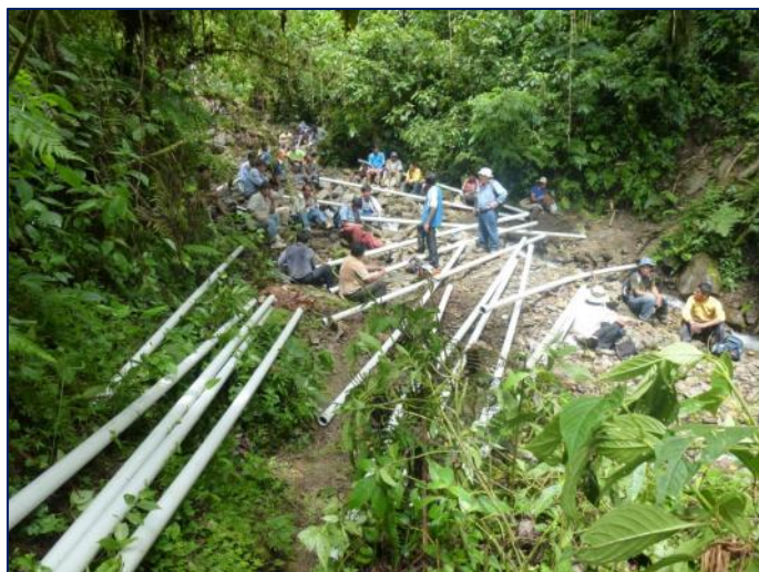
Members of the San Jose community help to place the pipelines, as part of their counterpart labor.
