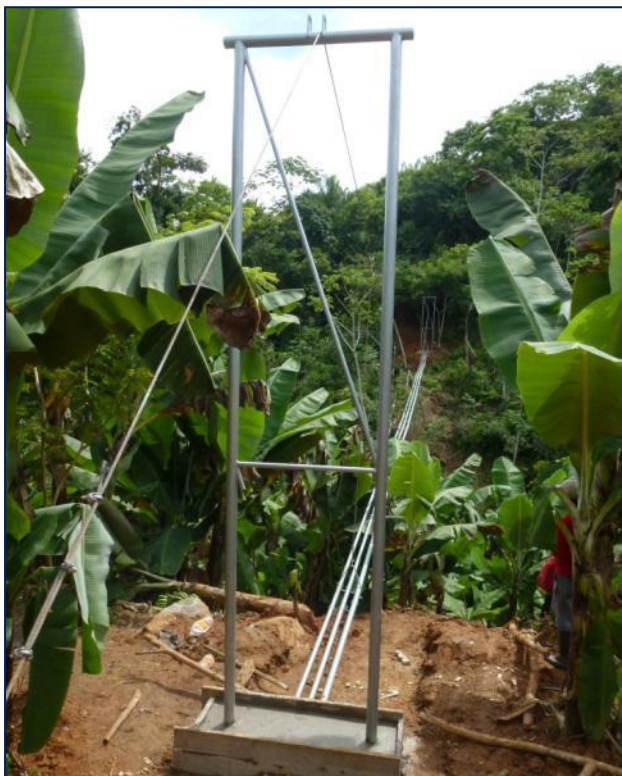
One of the pipeline bridges for the Alto Remolinos potable water system.
