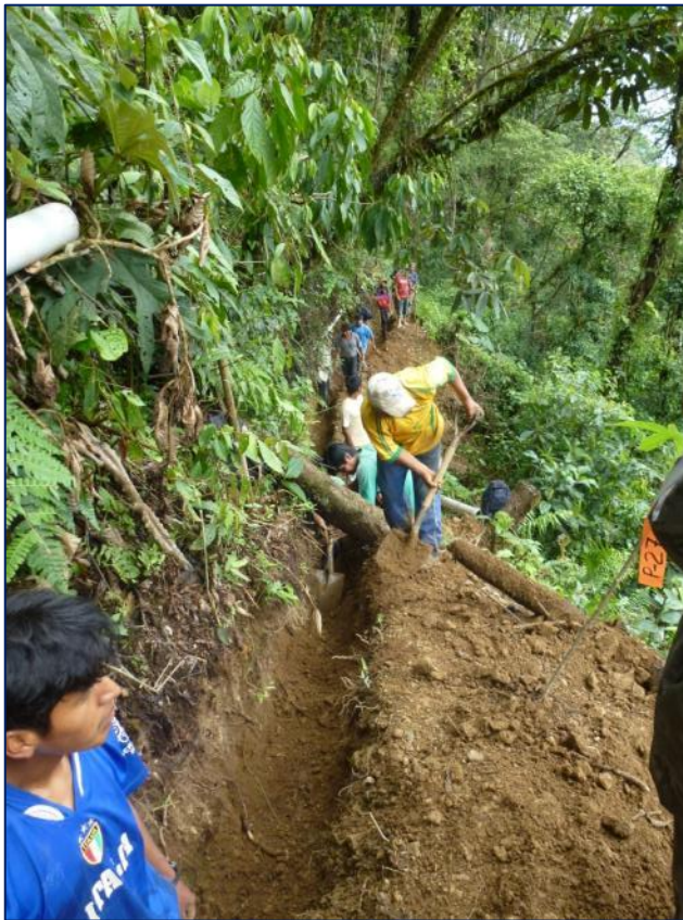
Counterpart labor: digging ditches for pipelines in Villa Camacho for the San Jose potable water system.
